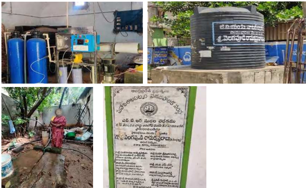
Photos 3. Water Kiosk infrastructure Mustapha colony: RO candles, storage, sump and foundation stone (by the Author).
