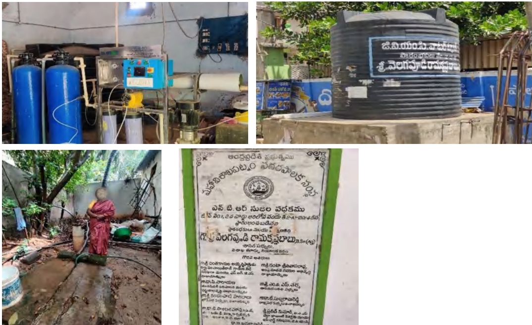
Photos 3. Water Kiosk infrastructure Mustapha colony: RO candles, storage, sump and foundation stone (by the Author).
